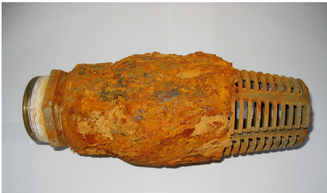
Figure 2.6.2. Figure showing severe galvanic corrosion on one-way valve where the house is made of Cast Iron with connector and sieve made of Bronze. (Photo by A. Einarsson).
