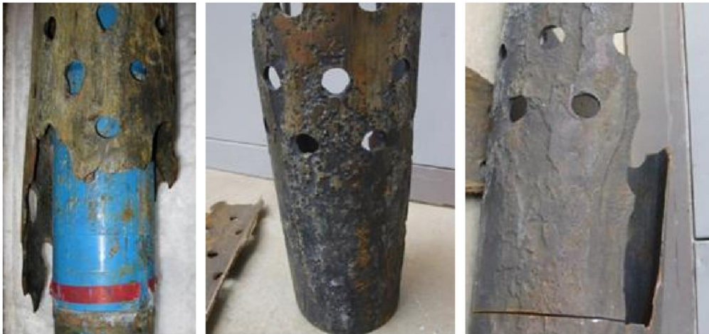
Figure 2.2. Pictures showing severe corrosion of well liner in the Krafla geothermal field well KJ-39. Corrosion of well liner at a blending point between HCl containing dry steam from lower geothermal system and wet fluid from upper system.
