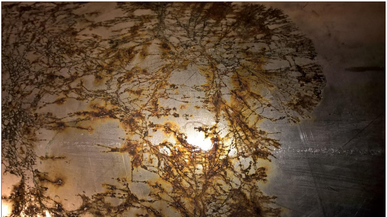
Figure 2.5.1. Stress corrosion cracking on the outside of a pipe from AISI 316 stainless steel (Photo Thorbjornsson).
